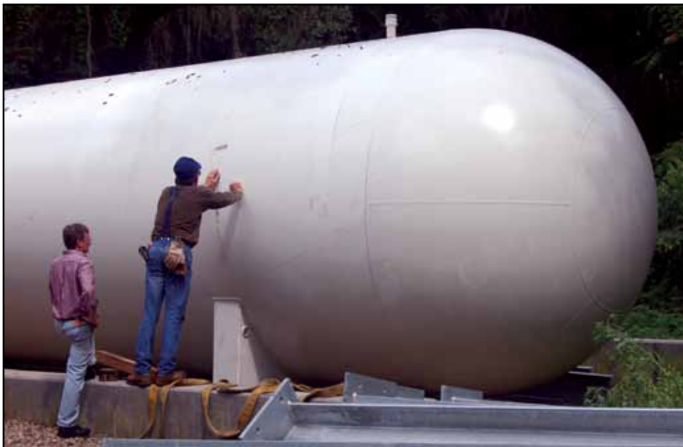
Maintenance and Construction Superintendent Richard Brooks supervised the unloading process when several semi trucks showed up on a muggy summer day to deliver the lab's four new helium tanks. The tanks will make pressurizing, storing and reusing the lab's costly helium supply easier. Photo by Amy Mast
